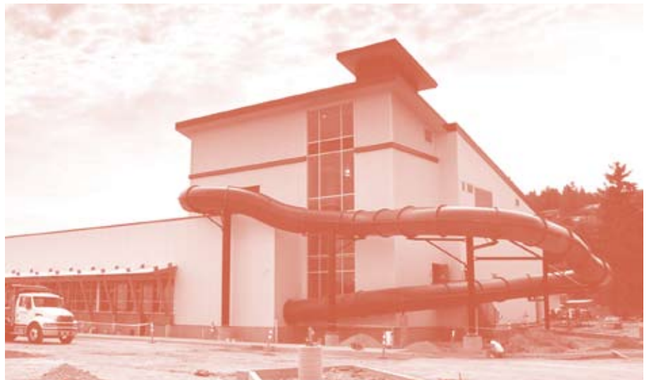
Workers put the finishing touches on the new Aquatic Centre, opening Oct. 24.
