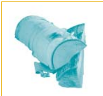
▲ Look for checks and cracks at the ends.
